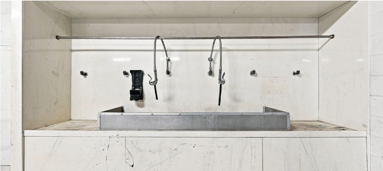
Plumbed wash station and workbench wall
